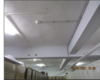
Photo of fire safety equipment smoke detector.JPG
