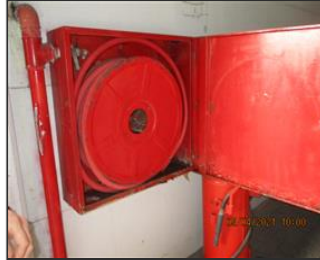
Photo of fire safety equipment fire equipment.JPG
