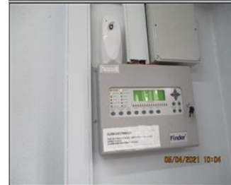
Photo of fire safety equipment fire alarm system box.JPG
