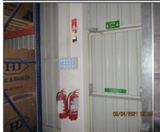
Photo of fire safety equipment fire extinguisher and emergency exit.JPG
