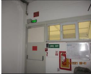
Photo of fire safety equipment fire equipment and emergency exit.JPG
