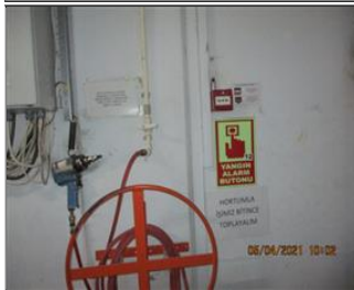
Photo of fire safety equipment fire alarm system.JPG
