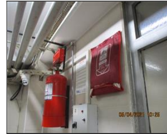
Photo of fire safety equipment fire equipment (2).JPG
